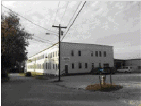
Abandoned maple syrup manufacturing facility with contamination issues including lead in soil and petroleum in soil and groundwater.
