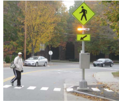
Rapid Flashing Beacon in Hanover, NH
