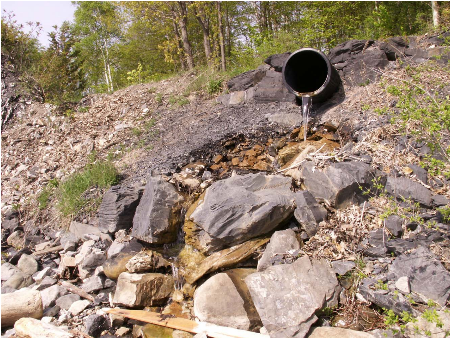
Perched culvert erodes the shoreline
