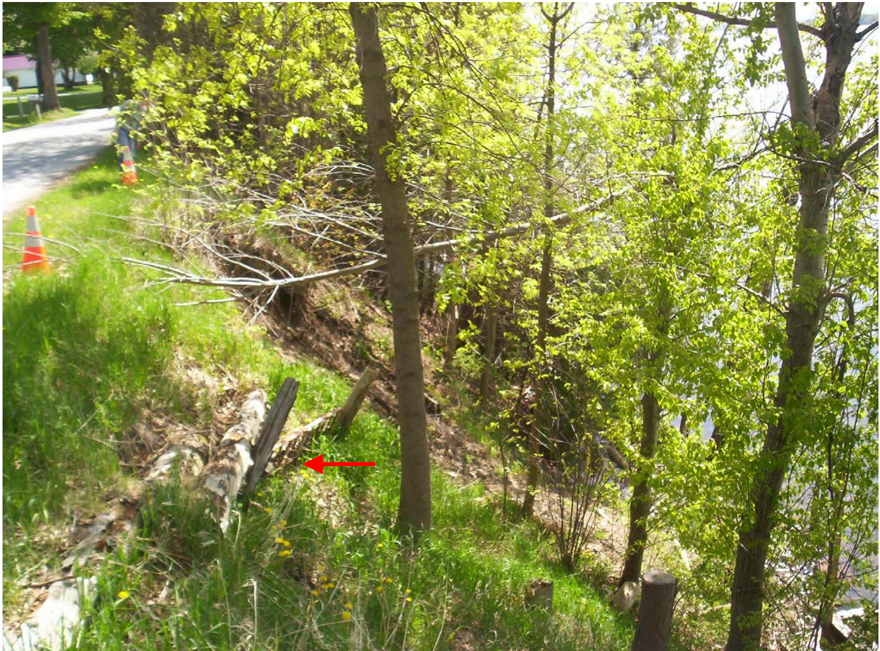
Soil creep is visible in the foreground where the stakes are no longer vertical
