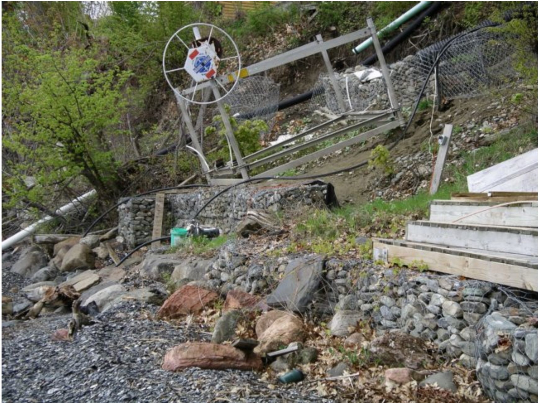
Successive attempts at erosion control. What is causing the erosion?
