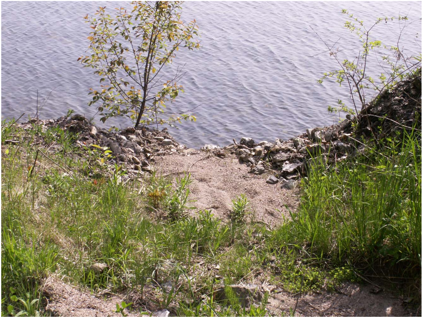
Rock fines at the road's edge indicate concentration point for stormwater runoff
