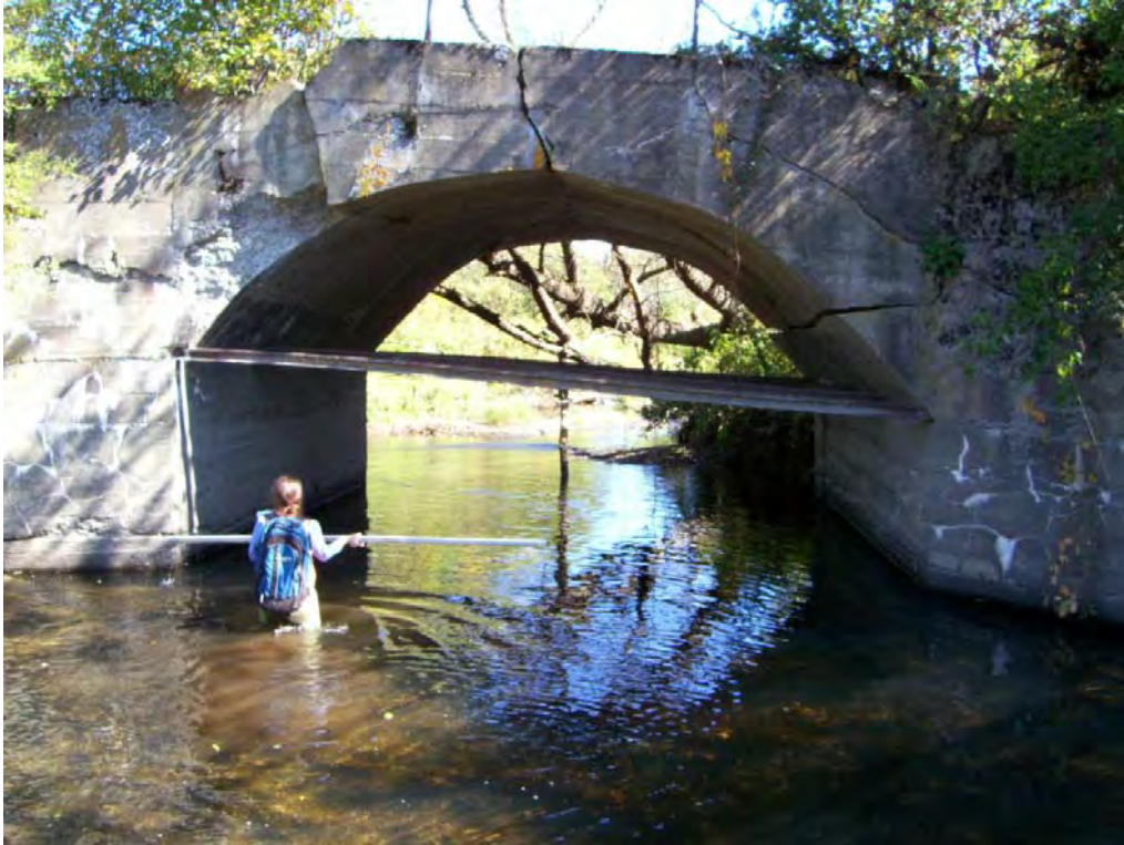
Figure 14. Farm bridge in reach RI5.01-A that is structurally unsound and is causing localized geomorphic instability.
