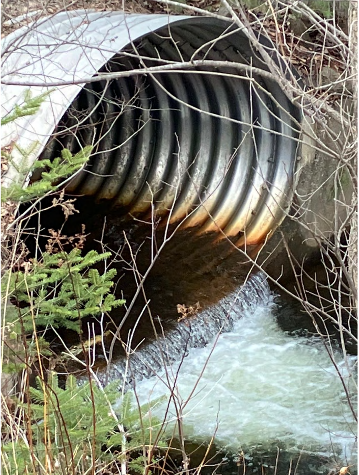
Culvert outlet slightly perched
