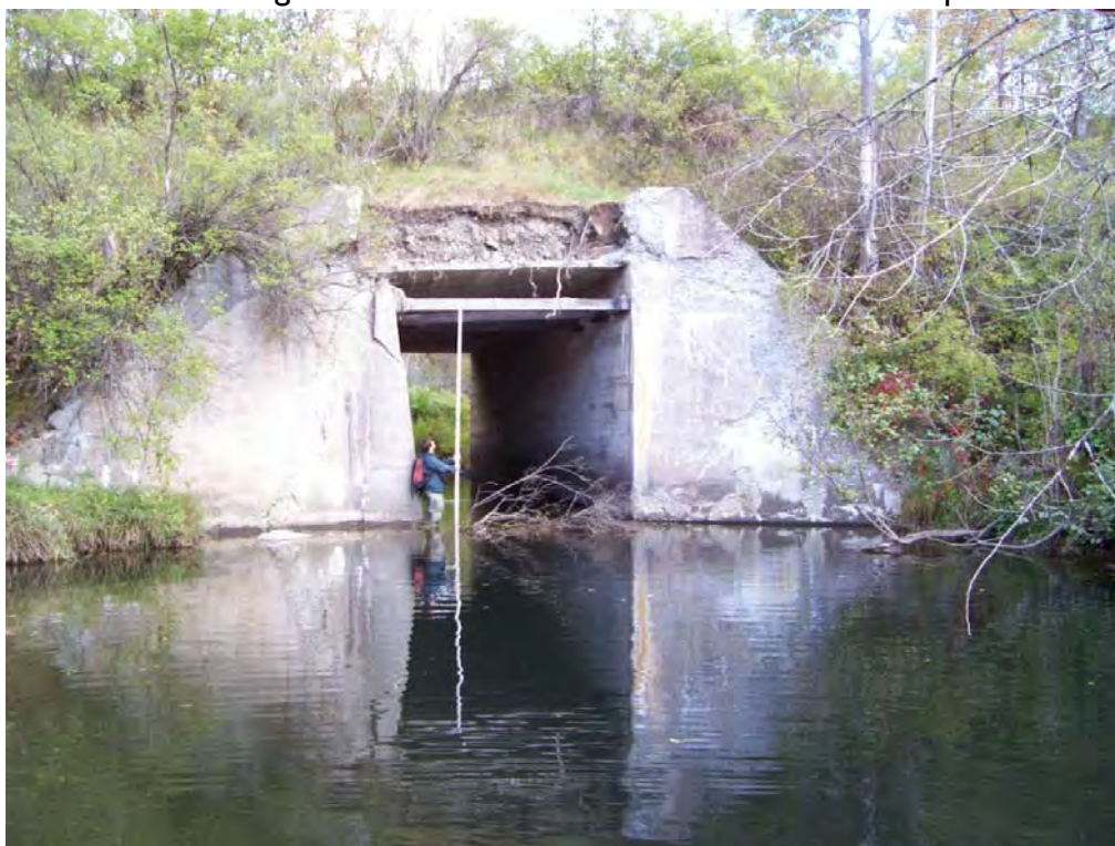
Figure 12. Rail to trail crossing in reach R15.02 has bank erosion above the outlet. This structure is undersized relative to the bankfull channel width and is recommended for replacement.
