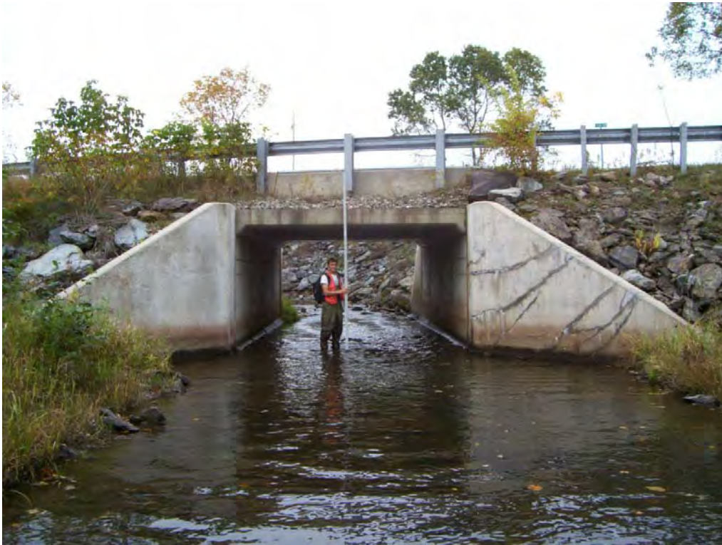
Figure 11. Bridge crossing at Frost Road within segment R15.05D. Centerville Brook approaches this structure at a sharp bend.
