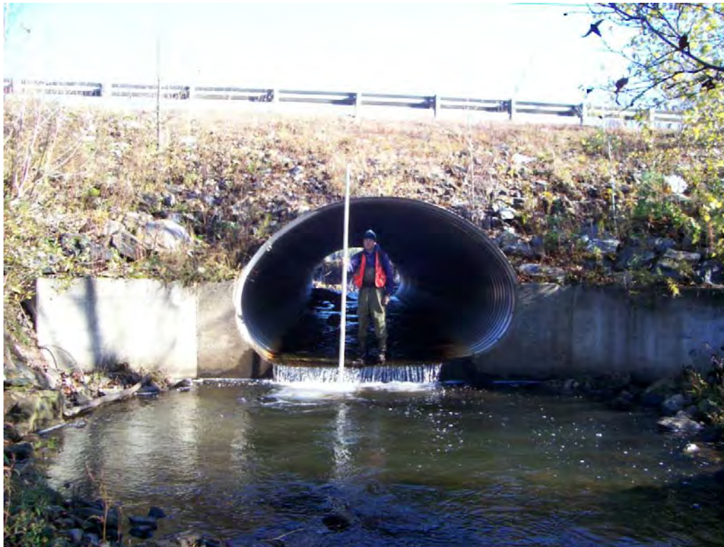
Figure 10. Culvert at Centerville Road in reach R15.07-B was flagged as “No Aquatic Organism Passage” using the Vermont Culvert Aquatic Organism Passage Screening Tool (Milone and MacBroom, Inc, 2008)
