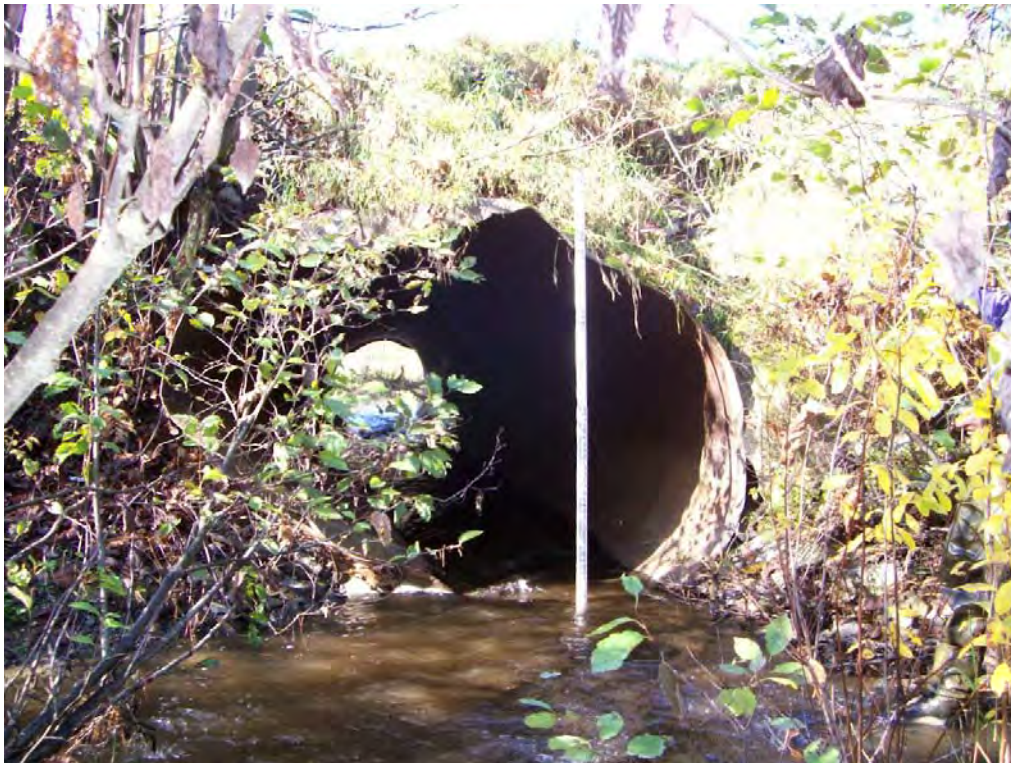
Figure 13. Brook Road culvert crossing in reach R15.07-A is undersized and impeding sediment transport. The culvert is in poor condition and has the potential to reduce AOP.
