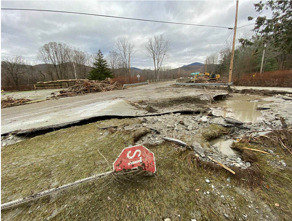
North Main and West Hill Road Following Halloween 2019 Flood
