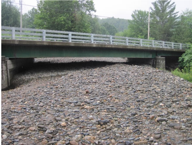
Figure 10. Sediment accumulation at West Hill Brook bridge.
