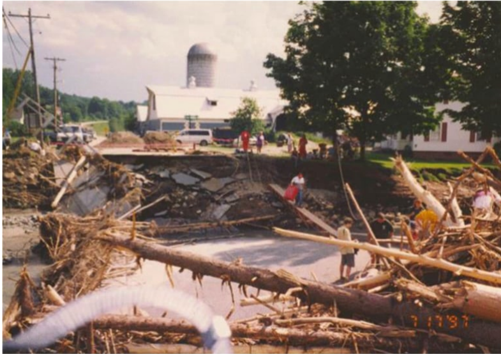
Figure 22. Looking south across the destroyed North Main Street Bridge following the 1997 flood.
