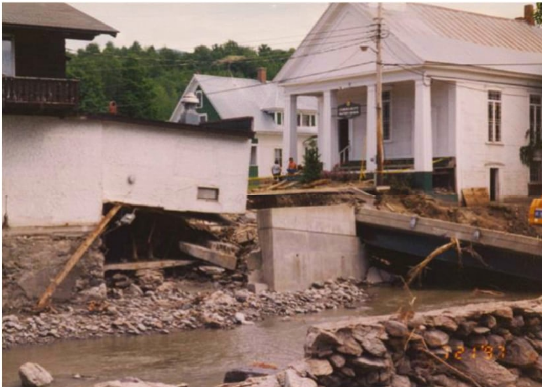
Figure 21. Looking northeast at the destroyed North Main Street Bridge in Montgomery Center following the 1997 flood.
