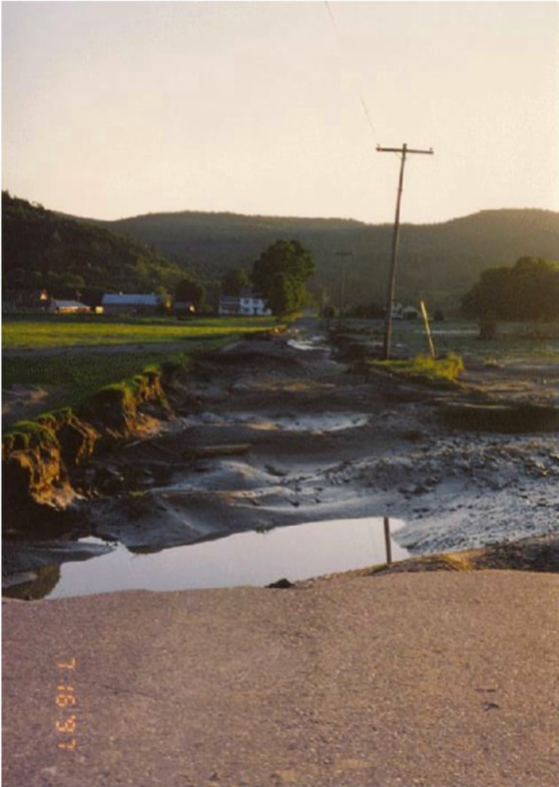
Figure 23. Looking west at damage to Longley Bridge Road following the 1997 flood.
