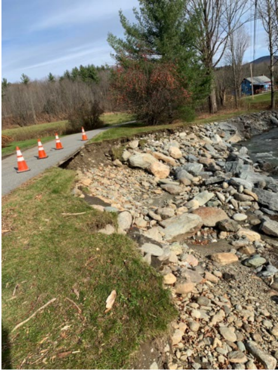
Brook Road Following Halloween 2019 Flood
