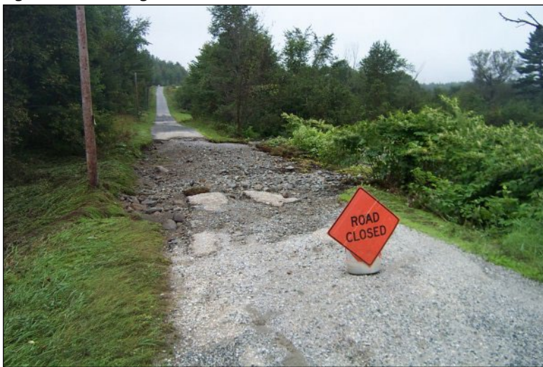
Figure 2: Flooding closes the Fanton Road
